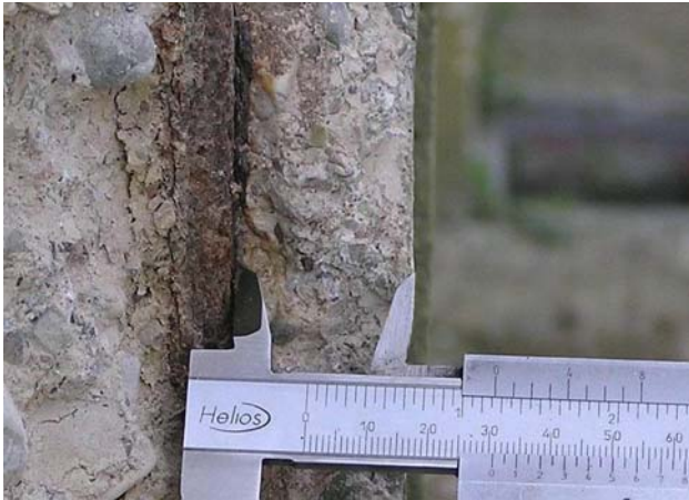
Fig. 3 Photograph showing a part of a structure where the corroded reinforcement increased its own volume forcing the removal of the concrete cover
